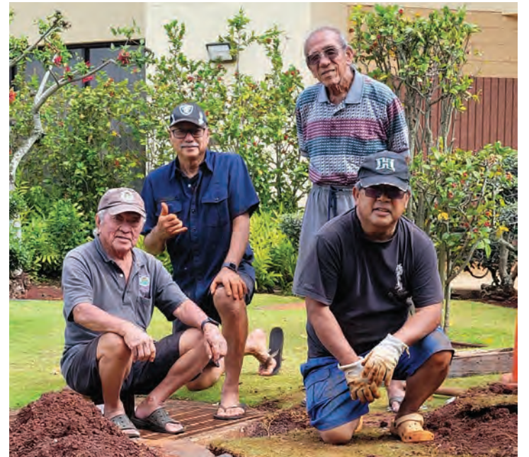
(L-R) Tom Nakamatsu, Glenn Awakuni, Paul Uyehara, and Craig Tobara working on the new drainage system.
